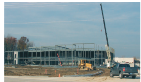
Construction began on Valenite in October as the cold winter days rapidly approached. Crews work from dusk-til-dawn to enclose the building before the snow flies.
